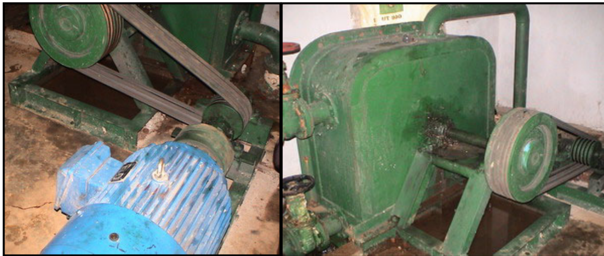
Figure 25: Turbine-Generator Connection through Belt, Ratnapura, source: Author
