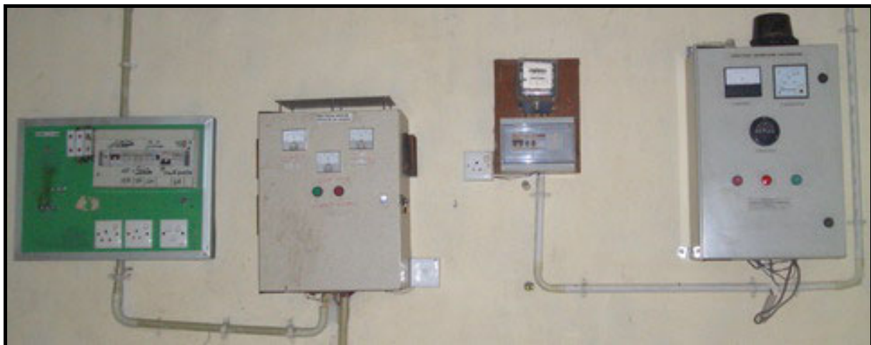
Figure 30: Controls and Switchgear of a MHP Plant in Ratnapura, source: Author
